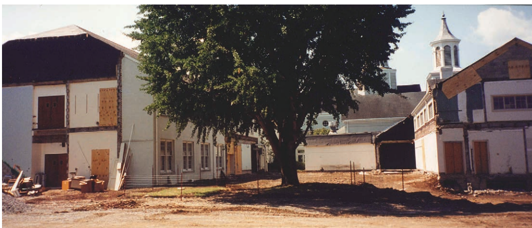
Construction of the office and Mothers' Day Out entrance around the gingko tree, 1999
